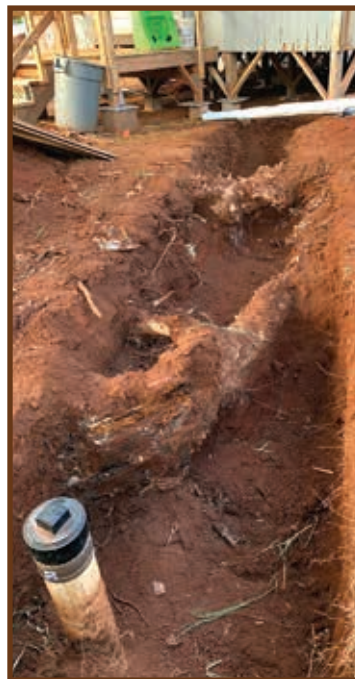
Cook Pine root intrusion
