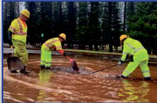
Elton Atacador, Norraine Pascua, and Henry Costales, Lāna'i Highways Division, clear clogged drains.
